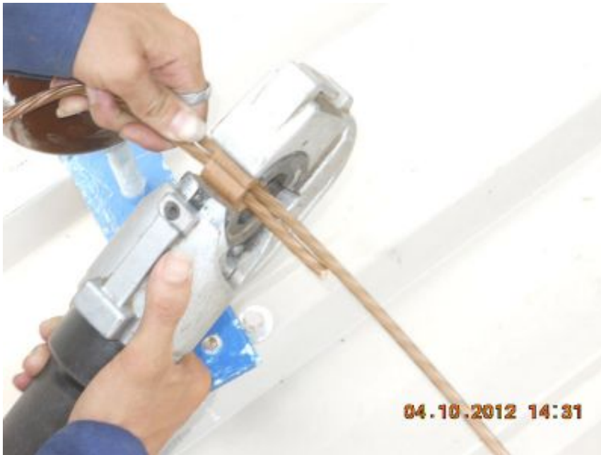
PICTURE OF INSTALLATION OF FM200 CLEAN GAS FIRE FIGHTING SYSTEM
