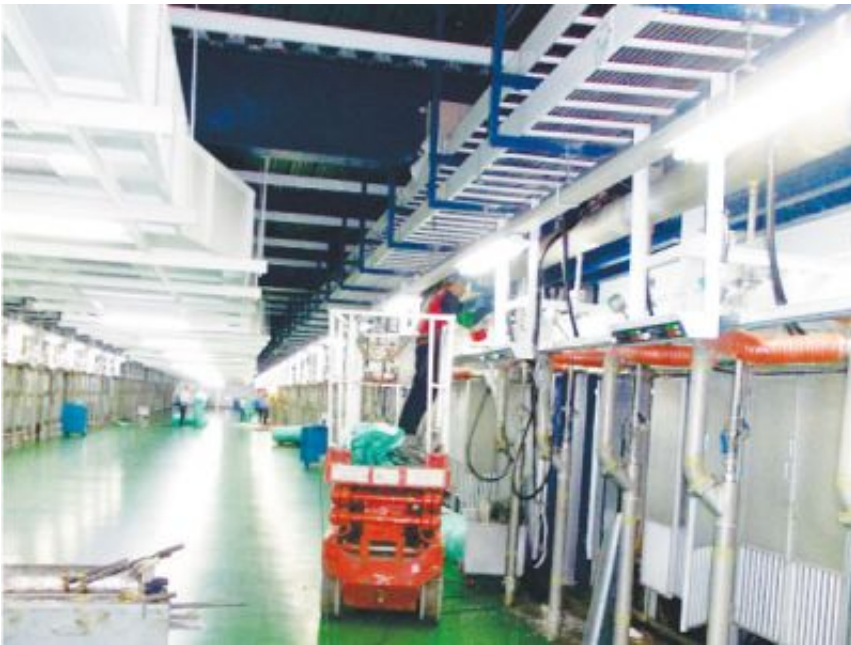
PICTURE OF INSTALLATION OF THE FACTORY LIGHTING SYSTEM
